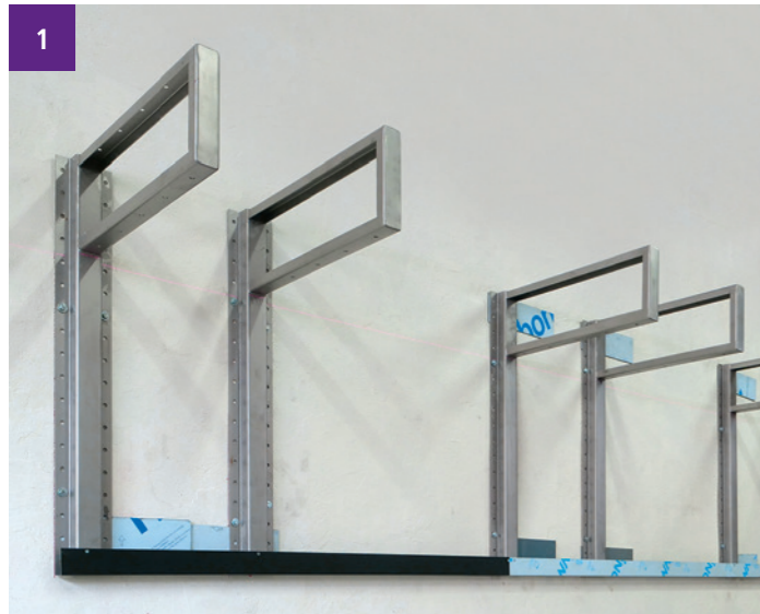
1 The layout of the rails marked beforehand (laser or tracing line) must match the layout diagram drafted by the architect.
