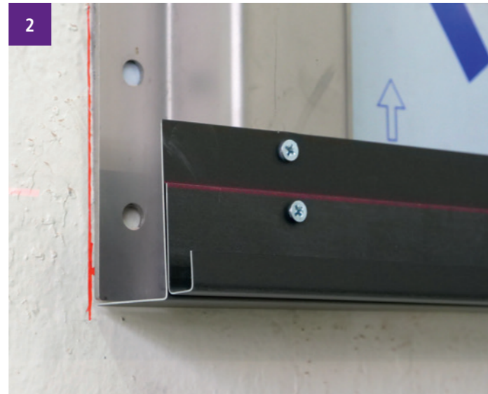
2 It is important to precisely align the bottom flashing to ensure that the cornice is completely straight.
